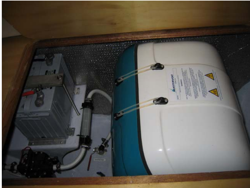
Genset installation under forward bunk.
